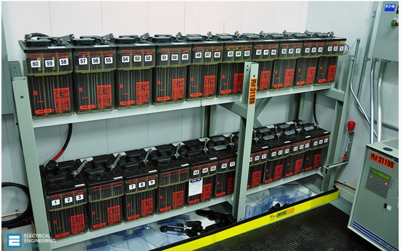
Substation DC Auxiliary Supply - Battery And Charger Applications (on photo: Newly completed DC auxiliary power supply of substation in Naramata BC; credit: Paul Chernikhowsky via Flickr)
