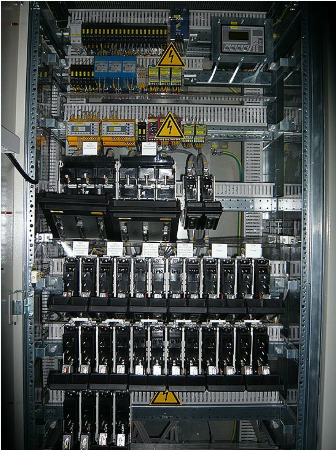
Auxiliary power supply switchboard (photo credit: bpa.ru)
