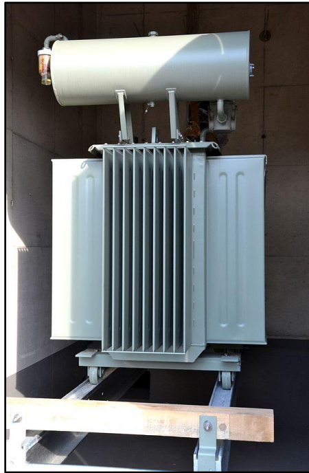
Fig.2.2: Oil transformer with air convection cooled heat exchangers in the front and at the side [8]
